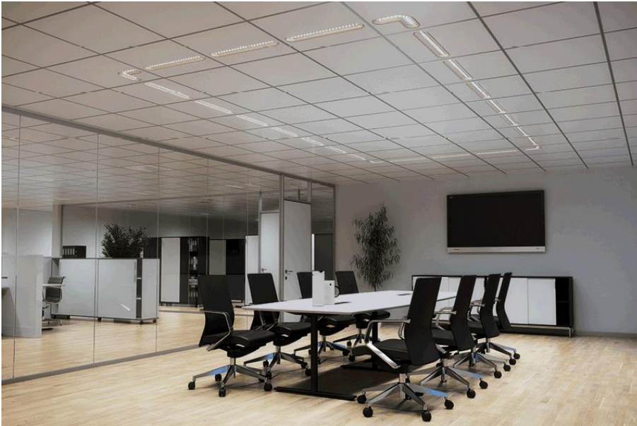
Photo of Riegens lighting project for office buildings
